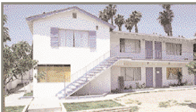
Prior to the redevelopment of Jeffrey-Lynne, buildings within the core suffered from years of neglect, including routine and preventative maintenance. Boarded-up windows, loose screens, and poor landscaping were common sites.
